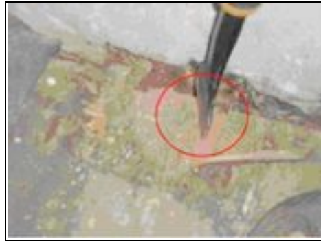
Wet rot, dry rot to floor
